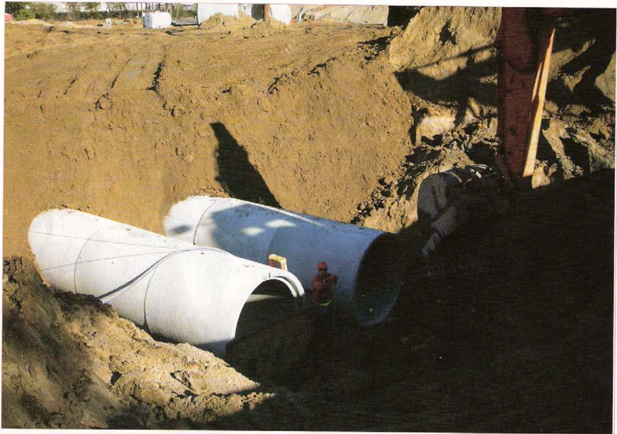
Today, Atlas Excavating Inc. performs sewer and storm sewer work, with water work on the side — specializing in deep 30- to 50-ft, wet or rock trenching. Occasionally, Atlas picks up some highway road reconstruction work, as long as there is a large amount of pipe work.
